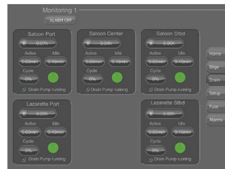
Example of a Pump Screen
